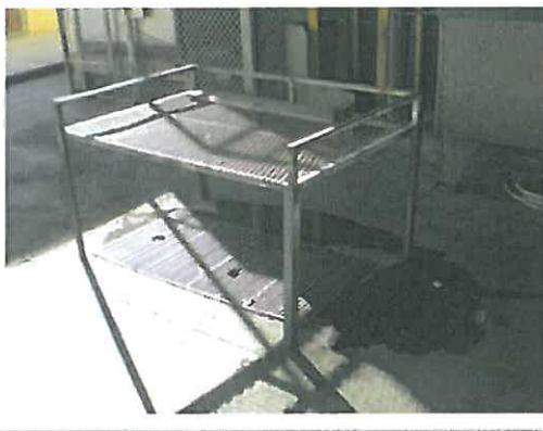
Fig 13 - Sump drain in Steam Clean area.
