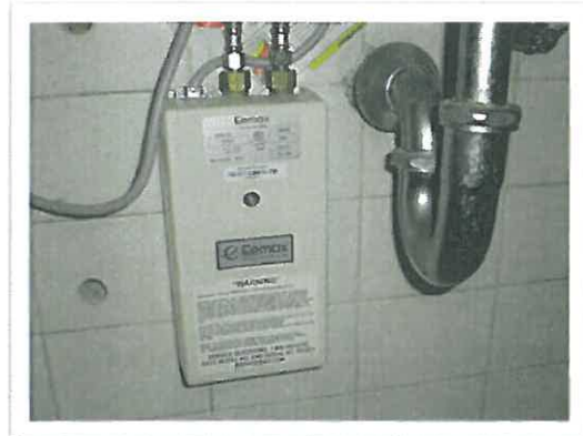
Fig 6 - Insta-hot water heater
