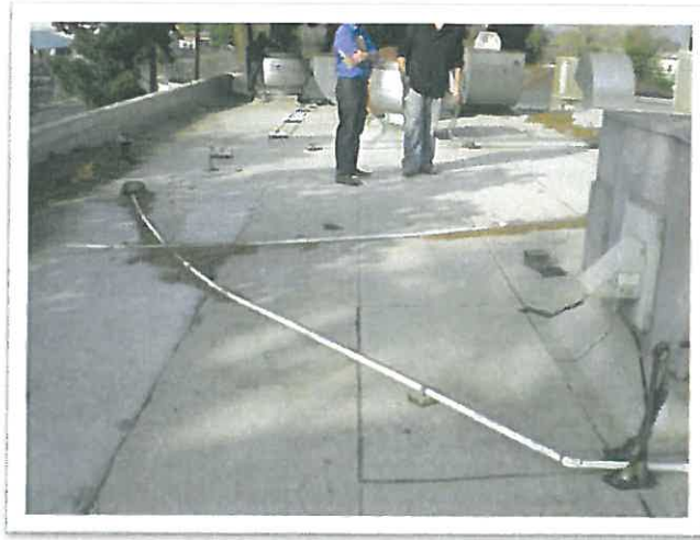
Fig 15 - PVC condensate drain pipe without adequate supports.
