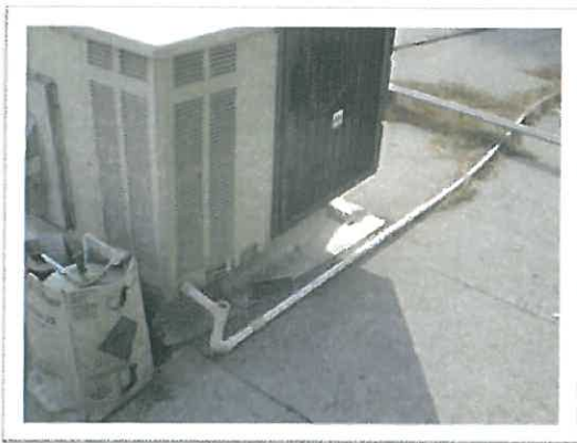
Fig 16 - Condensate drain without p-trap assembly.
