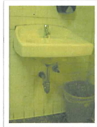
Fig 28 - Single temp lavatory at Men's restroom
