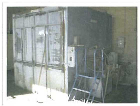
Fig 8 - Transmission washer in Steam Clean area
