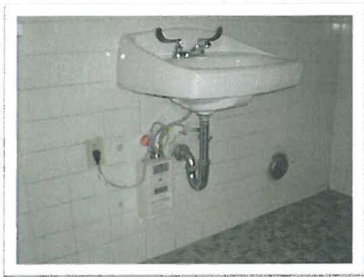
Fig 5 - Insta-hot water heater
