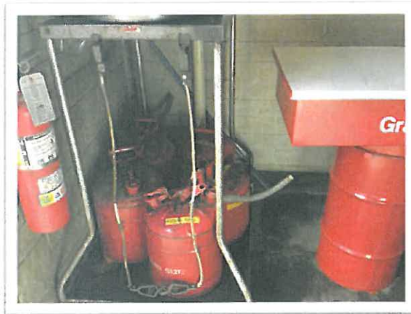
Figure M-4 - Fuel Storage Room 25
