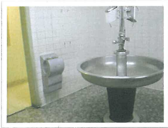
Fig 27 - Wash fountain in Men's restroom
