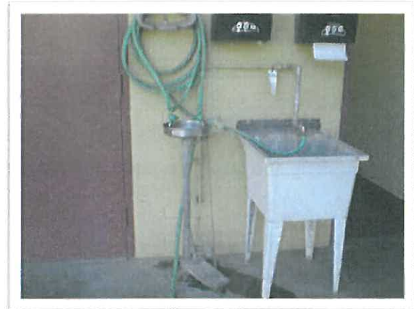
Fig 19 - Shop Building – obstruction around emergency equipment.
