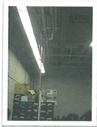
Fig 1 - Galvanized water pipe
