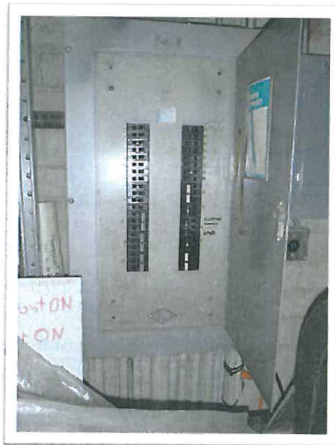
Typical Zinsco electrical panel
