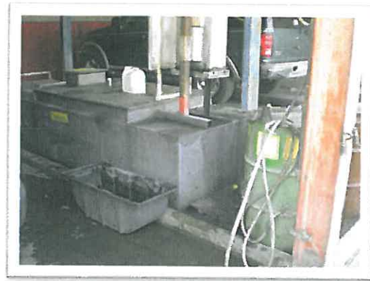
Fig 10 - Hose bib without vacuum breaker with hose laying on wetted pavement.
