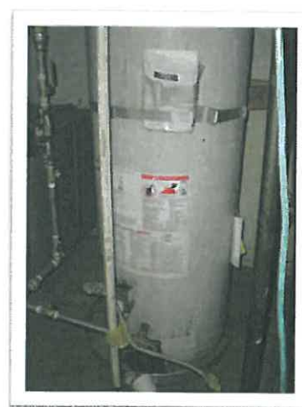
Figure 4 - Improper strapping of water heater
