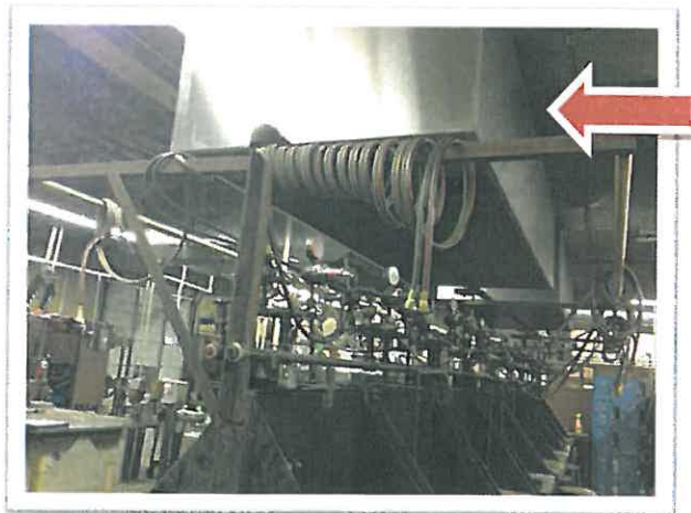
Figure M-1 - Updraft Exhaust Hood in Welding Shop 112B
