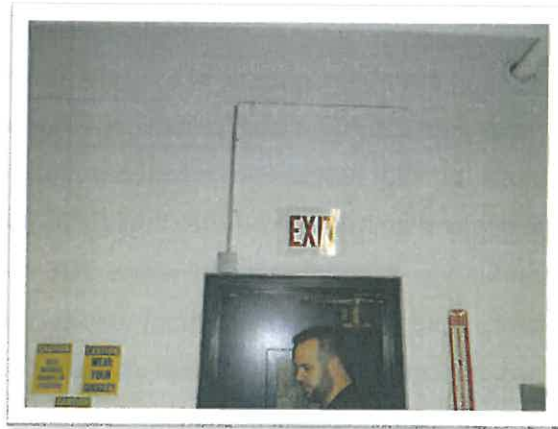
Exit sign should be replaced
