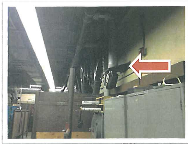
Figure M-2 - Local Exhaust Snorkels in Welding Shop 112B
