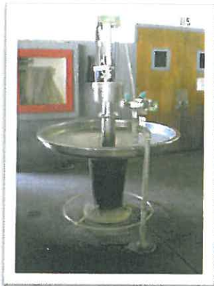
Fig 11 - No backflow or check valve on water supply of eyewash.
