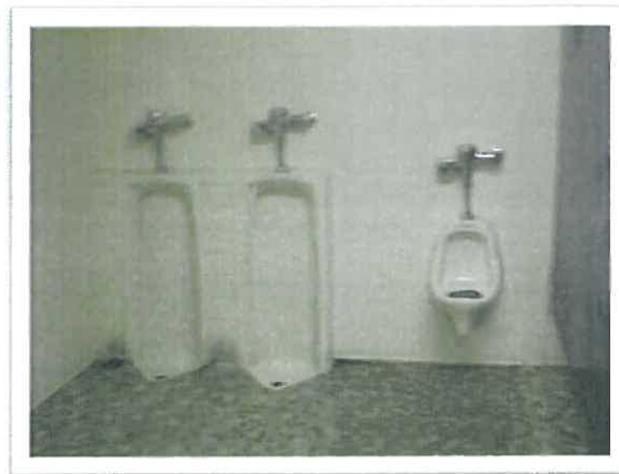
Fig 29 - Urinals at Men's restroom
